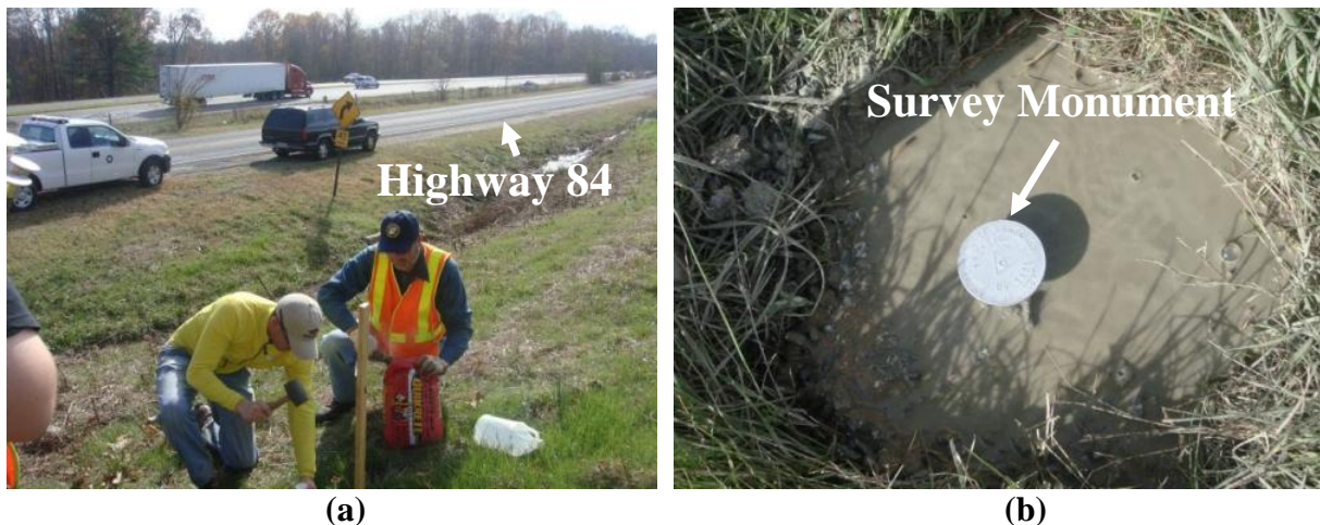
Figure 4.5. a) Installation of survey monument in the ground by UofA and AHTD personnel, and b) survey monument installed in the ground using Quickcrete®.
