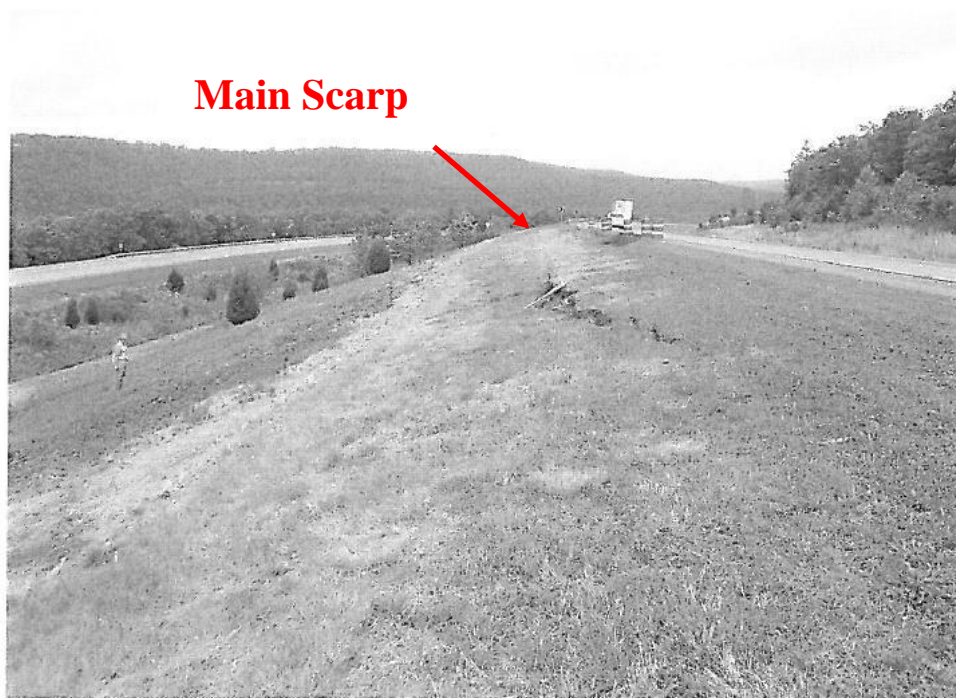
Figure 3.3. Looking north to the main scarp at the calibration site near Chester, Arkansas in May 2010 (from AHTD, 2010).
