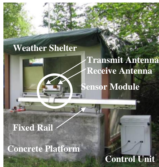
Figure 2.7. IBIS-L system at the Tessina landslide site (modified from Ingegneria Dei Sistem Online Brochure, 2007).
